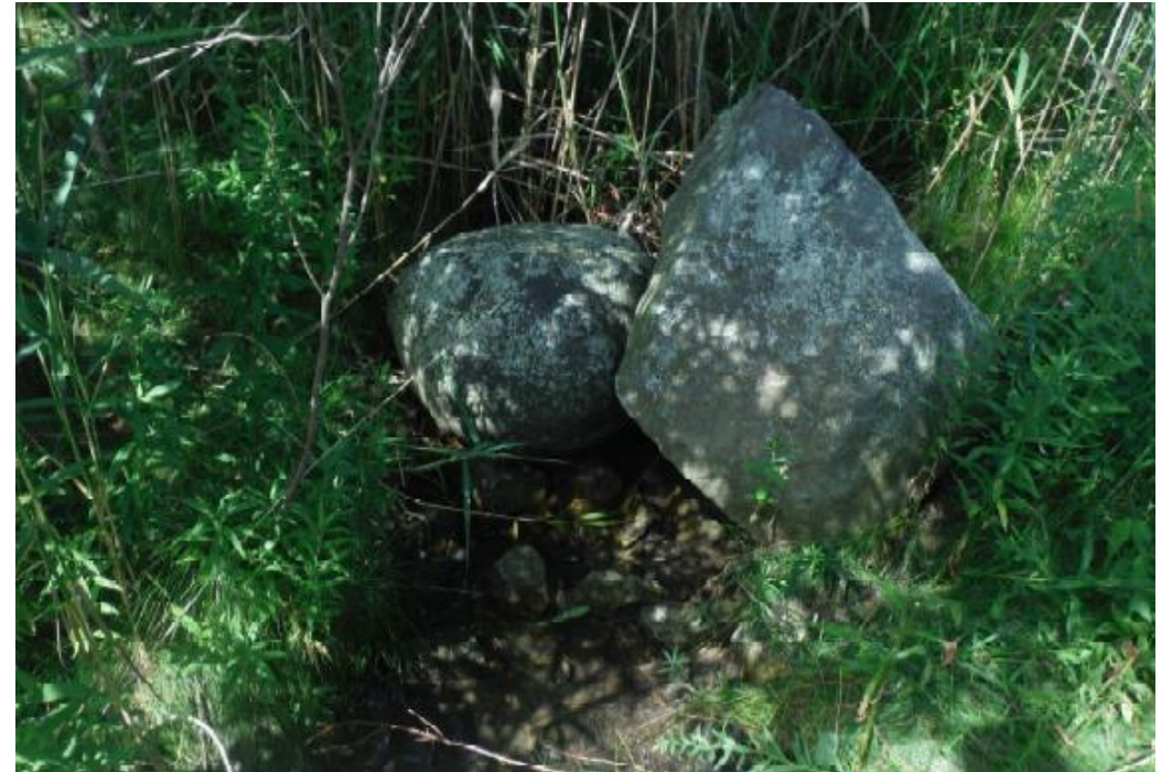
■ Rocks obstructing inlet pipe
