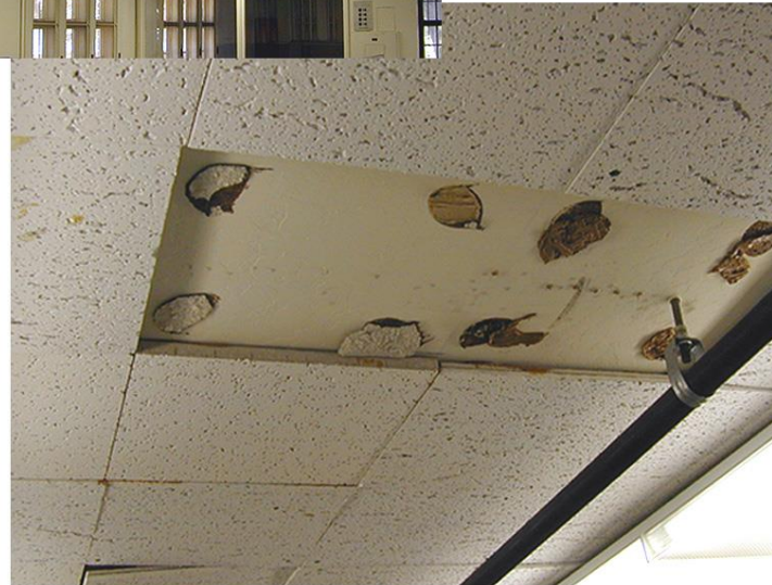
GLUE-ON ACOUSTIC CEILING TILE & EXPOSED BROWN MASTIC
